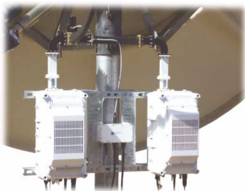
Redundant C-Band 5760 60 W high power SSPA system
